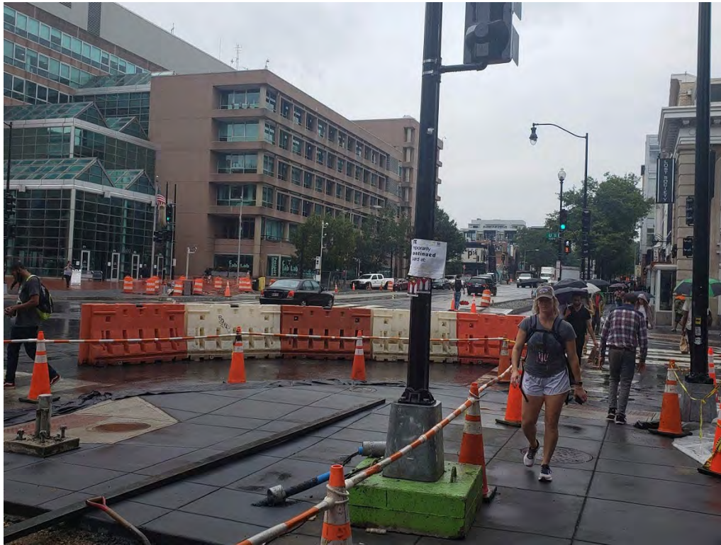
Completed sidewalk finish work at NEC of 14 th St. NW & U St.
