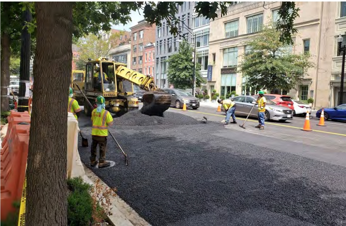
Placing & grading asphalt around MH covers before compacting SB lane of 1500 block of 14 th St
