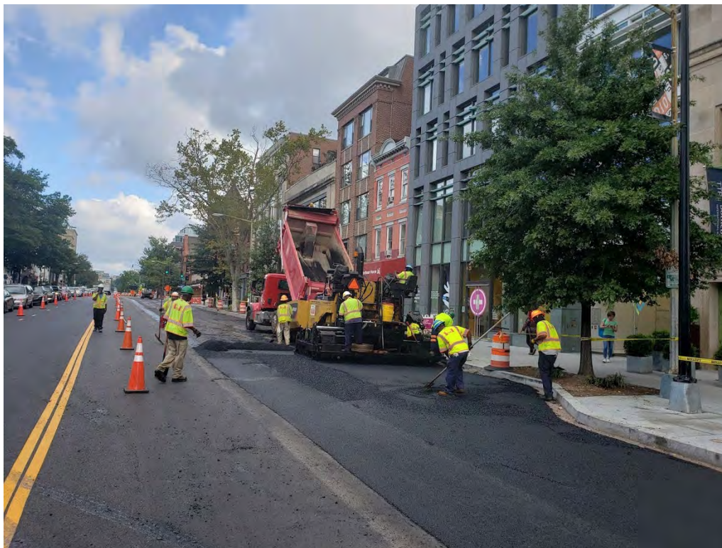
Paving operation along parking lane at 14 th St (NB) going towards P St.
