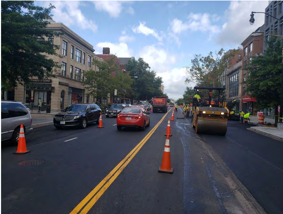
NB & SB lanes open with temporary markings installed as FMCC paved NB on 14 th St.
