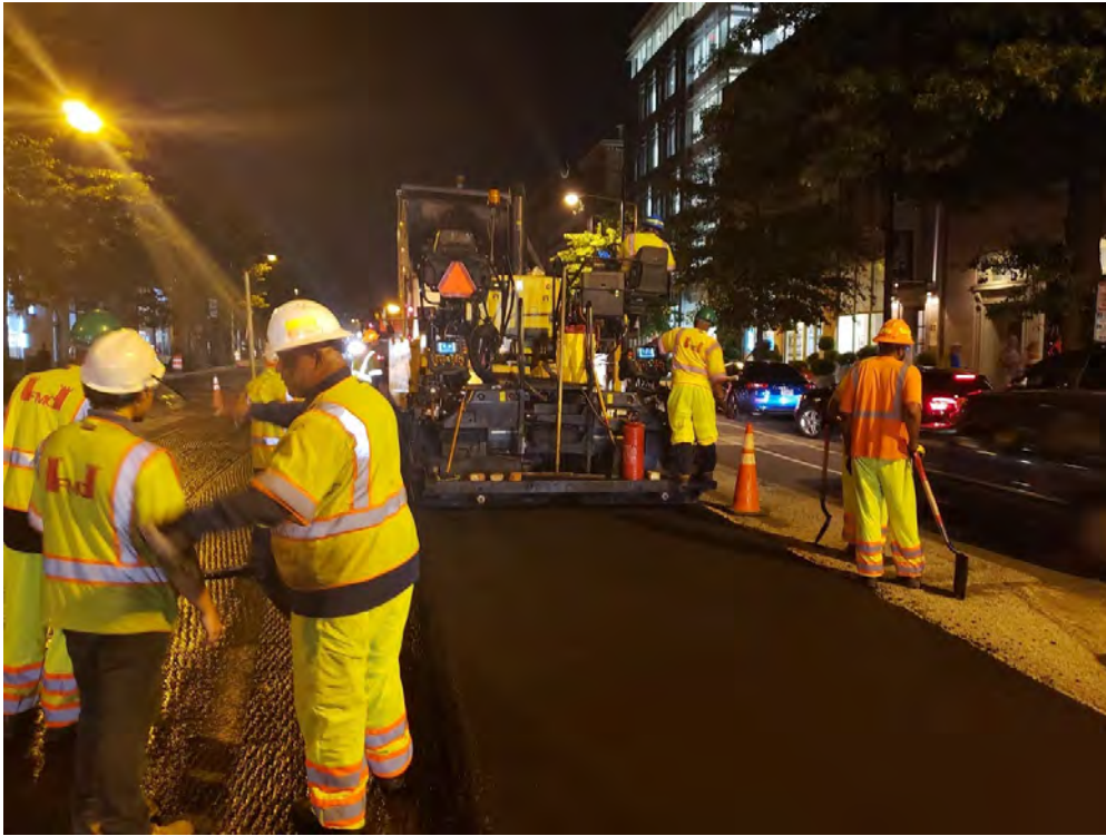
Night shift paving operations along 14 th Street from P to Corcoran St.
