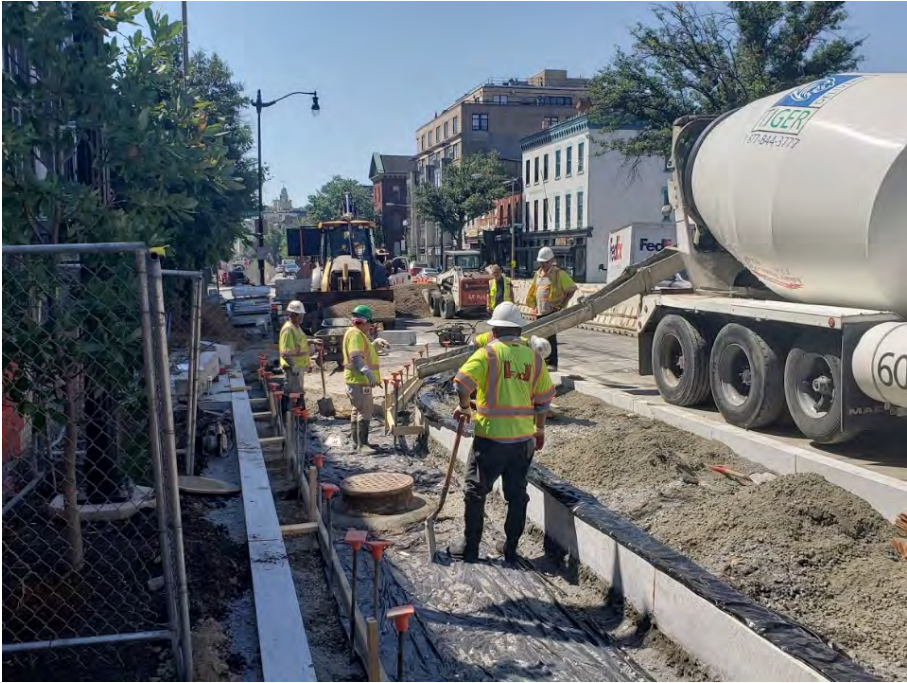
FMCC pouring concrete at bike lane near bus island near 14 th & R
