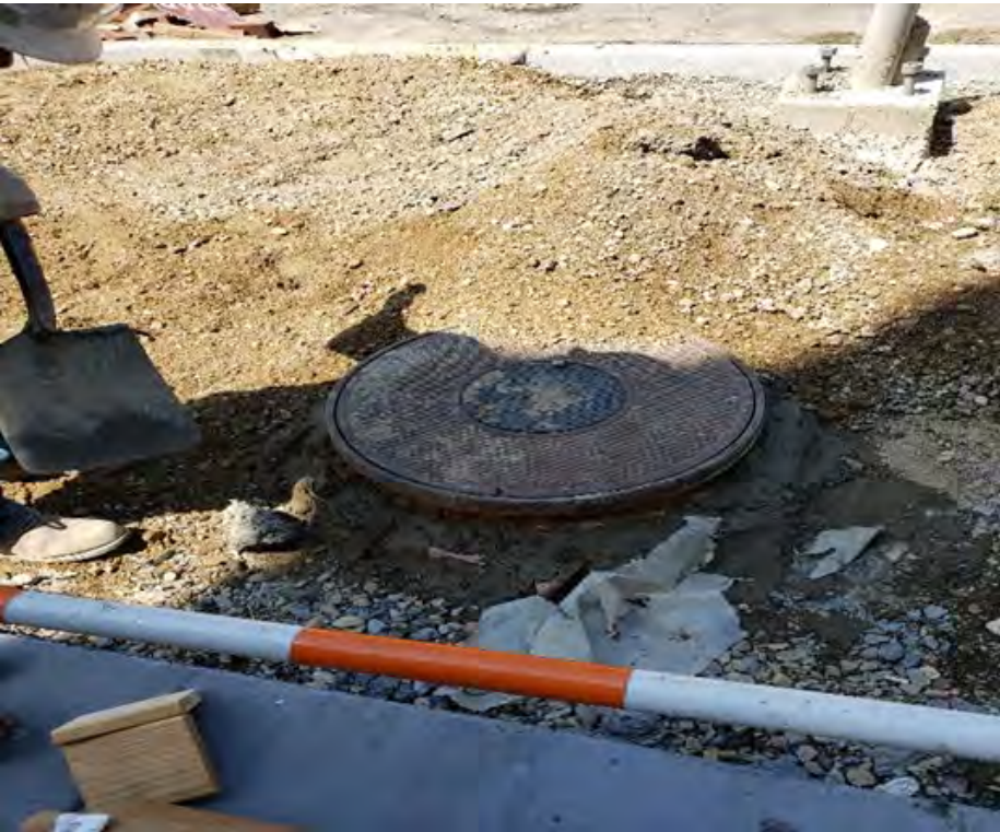
DEN vertically adjusted and raised two manholes near Wallach Place and 14 th St. NW
