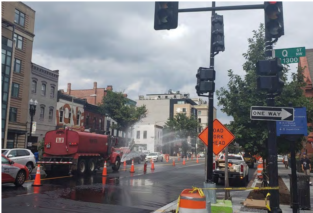
Cooling of asphalt on NB lane before opening up for traffic at 14 th St. NW & Q St.
