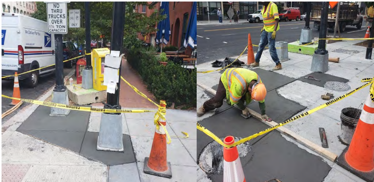
DEN completing punch list repair work at 14 th & P and 14 th St. & Q St. NW
