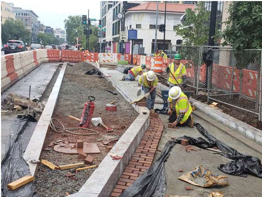
Brick gutter work for bus island at 14 th St. NW & R St. going NB
