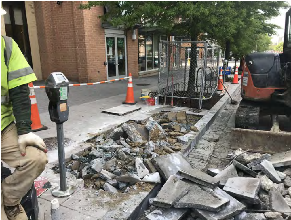
Excavating for installation of Fire Hydrant between V Street and W Street
