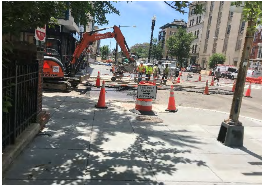
MOT set up for pedestrian crosswalk closure at the SEC of 14 th and Riggs St NW looking South on 14 th St.
