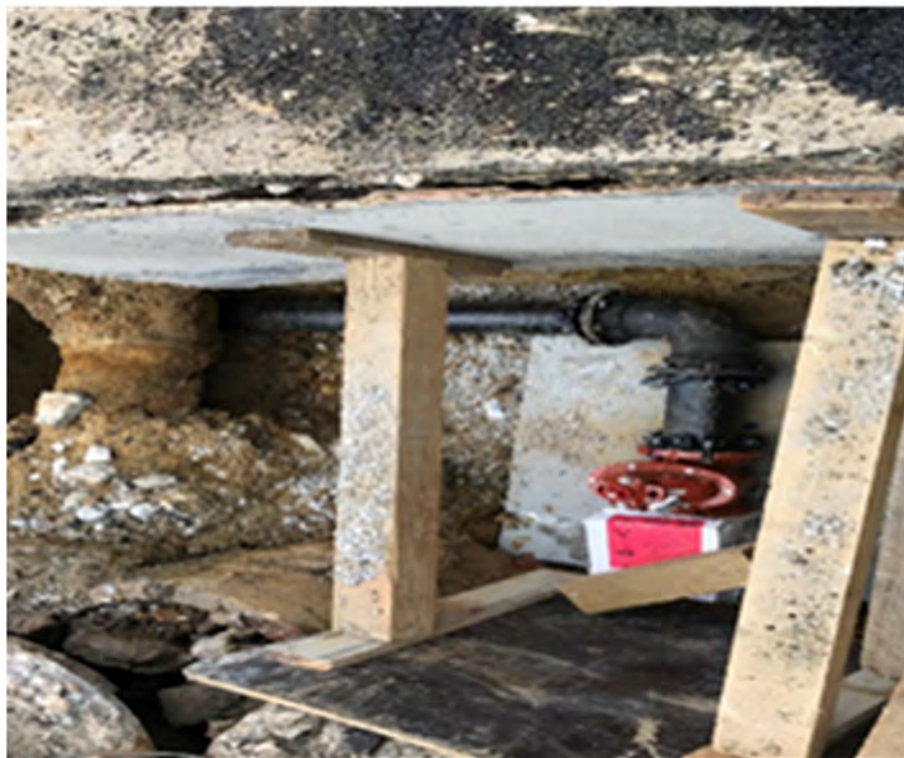
Progress picture for the fire hydrant connection at the SEC of 14 th St and S St NW.
