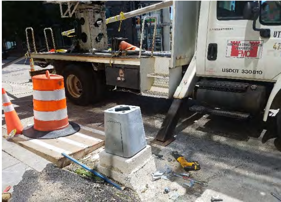
Transformer base installed at traffic signal TS-56.
