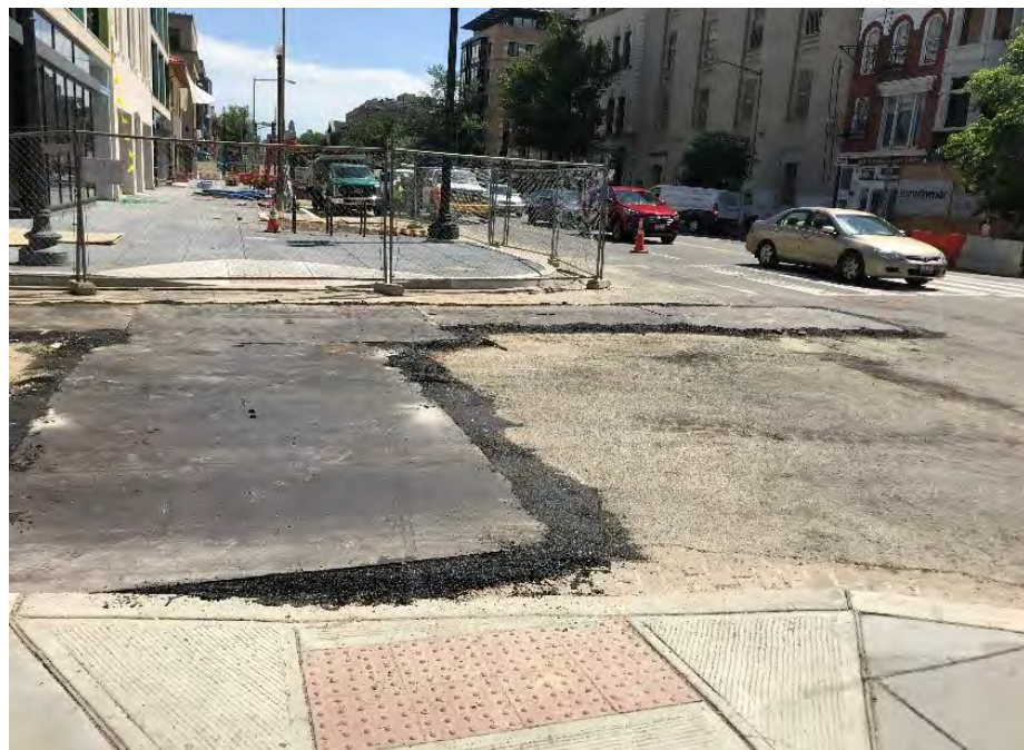
Putting back steel plates, pinning, welding and ramping with cold mix at the end of the shift
