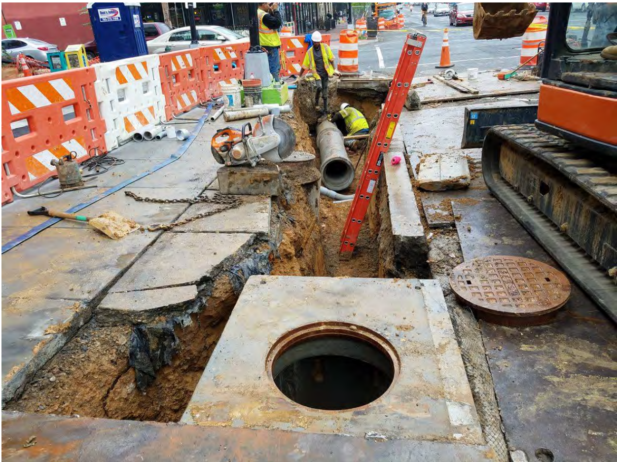
Installing the Connection pipe to Double Catch Basin at NEC of 14 th and P Street
