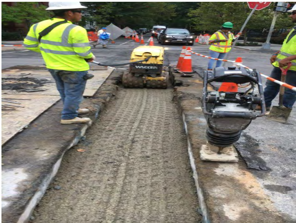
Abandon Street Car Track to be removed
