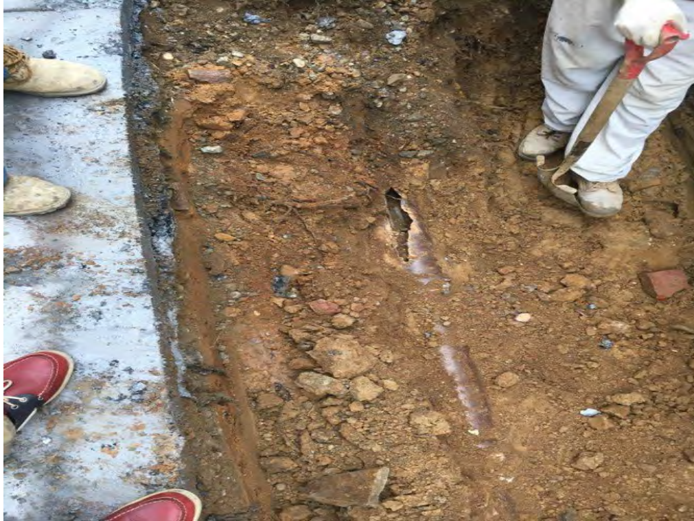
Unmarked Communication Cable found during excavation for CB-08
