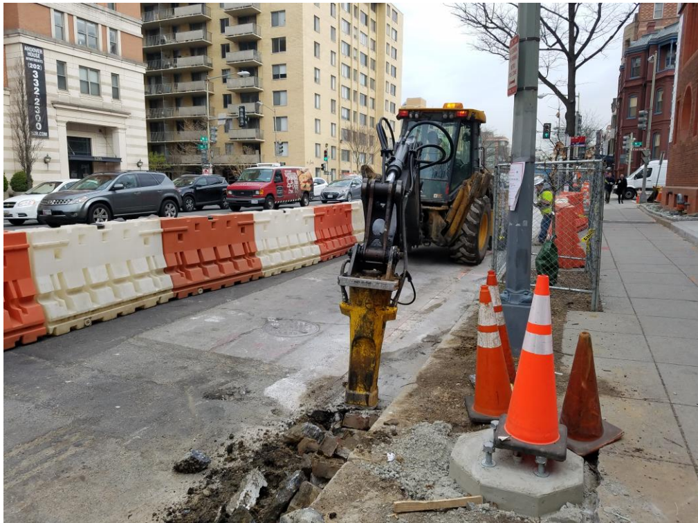
FMCC Demolishing the existing brick gutter between Thomas Circle and N Street
