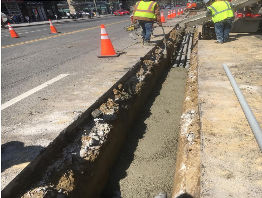
PVC Conduit encasement between Rhode Island and P Street
