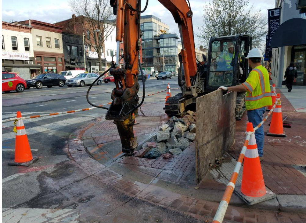
Demo of sidewalk for installation of manhole NE corner of Rhode Island Ave
